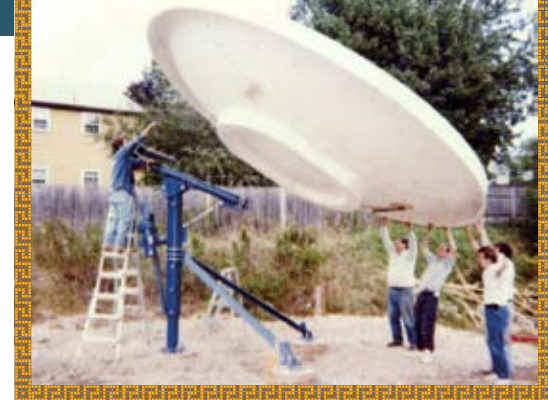
Moses (on the ladder) and an engineering crew install a down-link dish for Fox Network.
