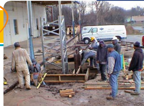
Workers prepare to pour the concrete base for KRYH-LP, 104.7 FM's tower in Temple, Texas.
